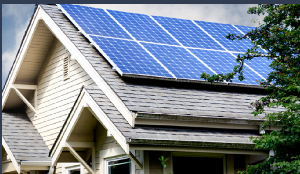
The County has inspired solar installations for 235 homes within the last two years.
